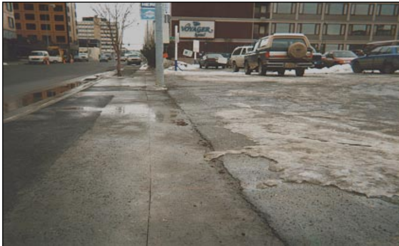
March 27, 1999. Sidewalks are wet from parking lots, some ponding along curbs (5th Ave.)
