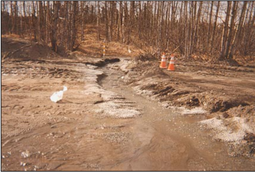
V-ditch to Infiltration Area from TU01
