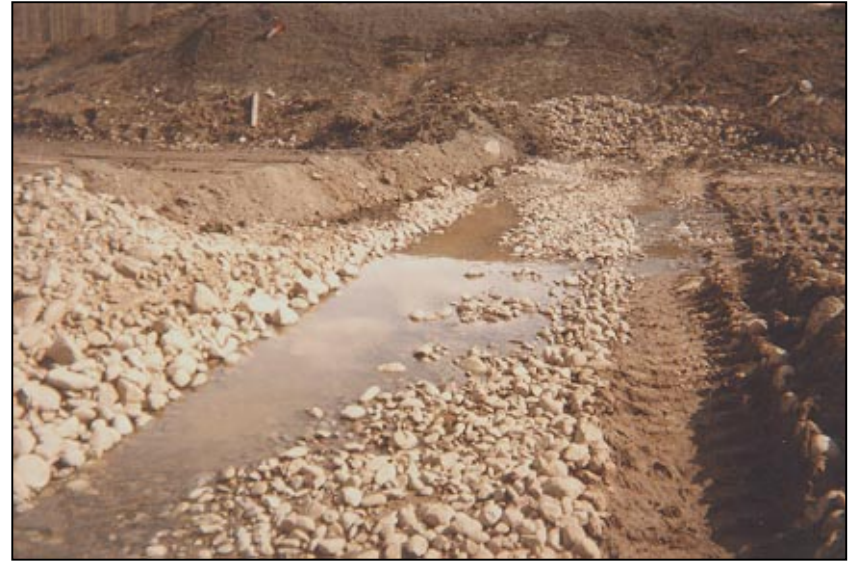
Berm Directing all Flow to Ditch (TU07)
