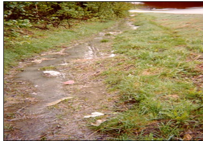
Turbid Flow to Culvert - Station MTV01
