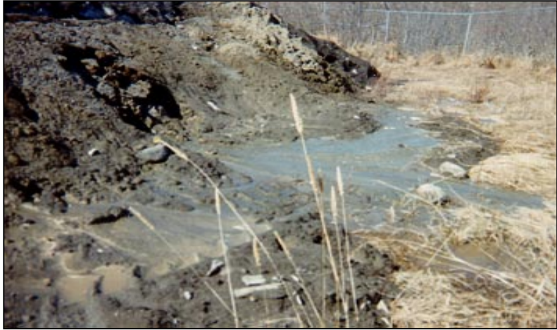
Berm Failure Above Pond (TU02) - (4/23/99)
