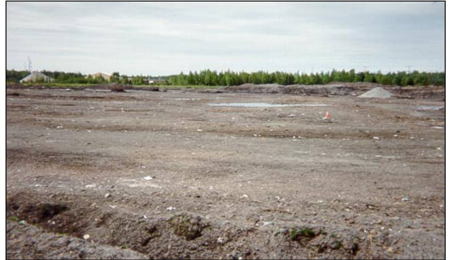
Minor Ponding in Middle of Site
